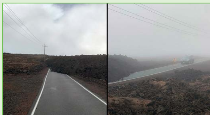
Lava covering the access road to the NOAA Mauna Loa Baseline Observatory during the 2022 Mauna Loa eruption
